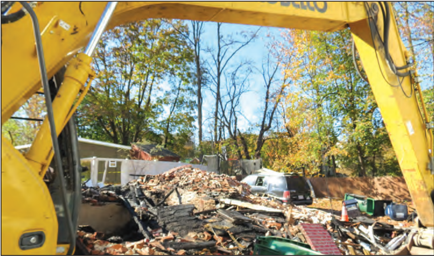
The rubble on Brick Row in Wappingers Falls in November 2023.
