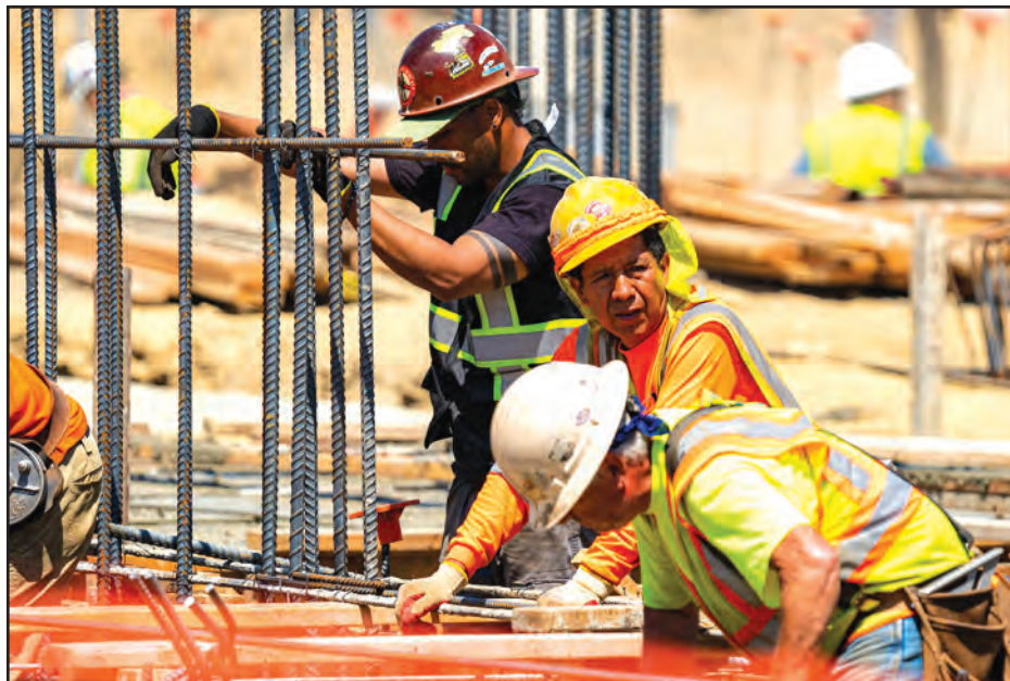
Workers begin construction on the "Phase Two" renovations at Heritage Financial Park, home of the Hudson Valley Renegades minor league baseball team. All construction is slated to be completed by opening day of April, 2024.
