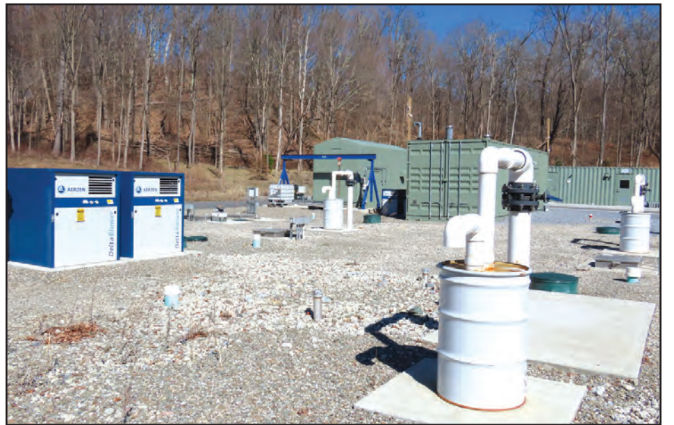
The wastewater treatment plant near the Inn at Historic Bellefield on Route 9 is fully functional and lines are planned to tie into sewer lines from the Town of Hyde Park near St. Andrews Road. Photo by Curtis Schmidt
