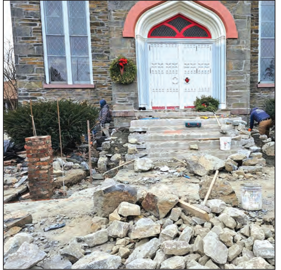
A ribbon-cutting ceremony to show the renovations at Zion Episcopal Church will be held on April 5 in Wappingers Falls. Pictured is work being done as the renovations were being completed.
