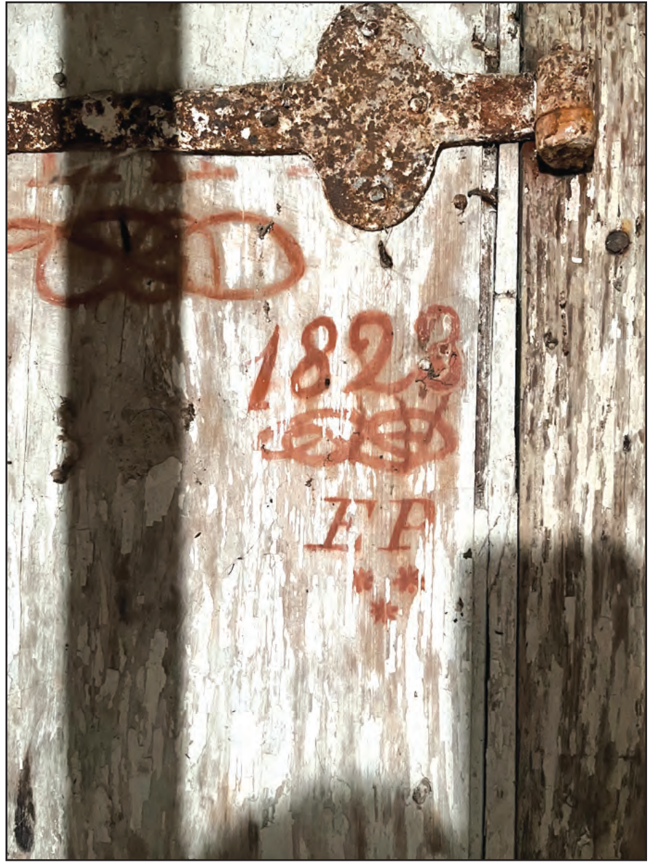
The basement door of the mystery historic house in Clinton: Tune in to the Clinton Historical Society's program on September 8 at 7:30 p.m. to find out whose initials those might be.
