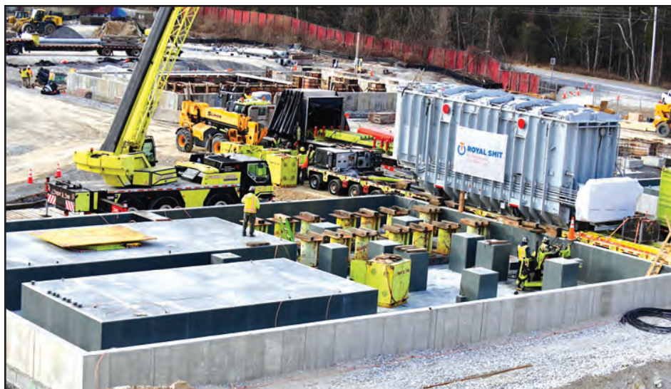
A specialized transformer called a phase angle regulator (PAR) is pictured on an oversized transport truck at the site of a new electric substation in the Town of Dover. Courtesy photo
